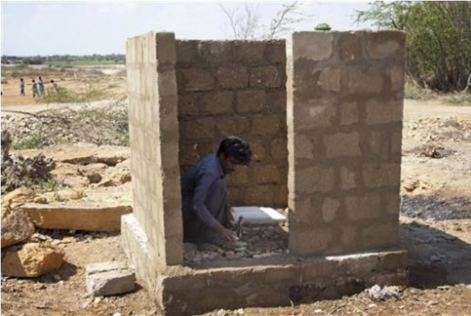
In this Tuesday, March 3, 2015 photo, a Pakistani worker constructs a toilet in Thatta, Sindh province, 100 kilometer (62 miles) southeast of Karachi, Pakistan. More than 40 million people in Pakistan do not have access to a toilet, forcing them to defecate in the open, which in turn is a major contributor to stunted growth in the country, a top UNICEF official said. UNICEF is working with the Pakistani government to improve sanitation by doing things like encouraging people to wash their hands more often and working with communities to help them build toilets. (AP Photo/Shakil Adil)
