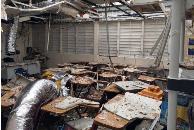
A classroom in Puerto Rico shows the damage from Hurricane Maria, which was a category 4 storm when it struck the US territory on September 20, 2017. Credit: Provided by Rosaura Orengo-Aguayo
