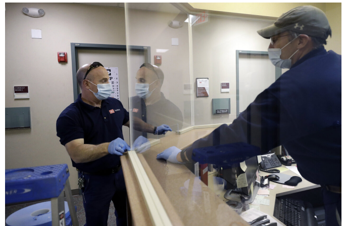
In this Wednesday, May 20, 2020 photo carpenters John Mackie, of Canton, Mass., left, and Doug Hathaway, of Holliston, Mass., right, apply trim to a newly installed plastic barrier in an office area, at Boston University, in Boston. Boston University is among a growing number of universities making plans to bring students back to campus this fall, but with new measures meant to keep the coronavirus at bay. (AP Photo/Steven Senne)
