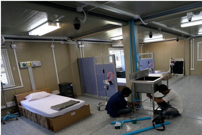
Workers install a sink at field hospital for COVID-19 patients at the 11th Army Region base in Bangkok, Thailand, Friday, July 2, 2021. As Thailand faces growing numbers of COVID-19 cases and related deaths during a devastating third wave of the coronavirus, there are concerns that it will face a shortage of hospital beds, intensive care units and ventilators for seriously ill patients. Credit: AP Photo/Sakchai Lalit
